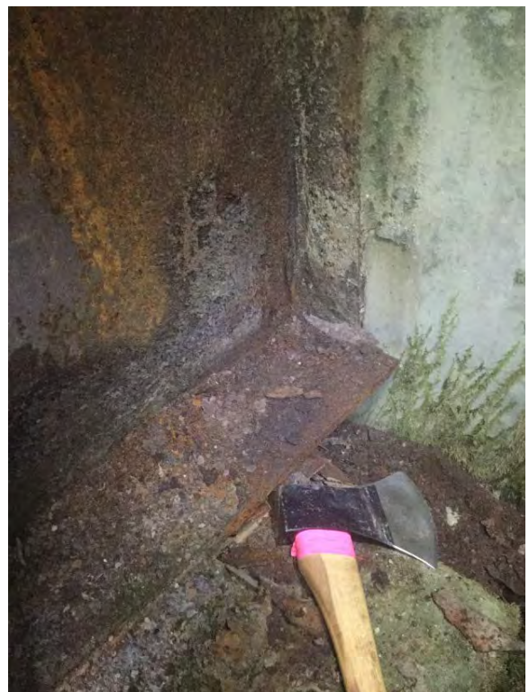
Right Bank Abutment when facing downstream - upstream side heavy rust scale at end of bridge
