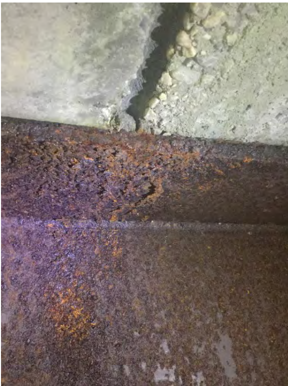
Typical rust scale at joint (upper flange)
